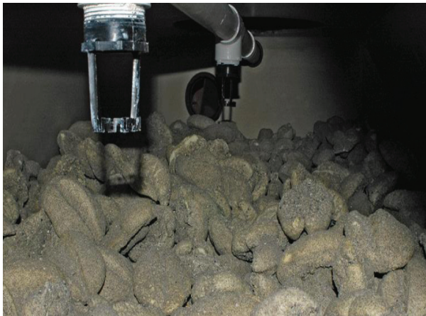
MetaRocks media bed and spray nozzles inside Eliminite tank.
